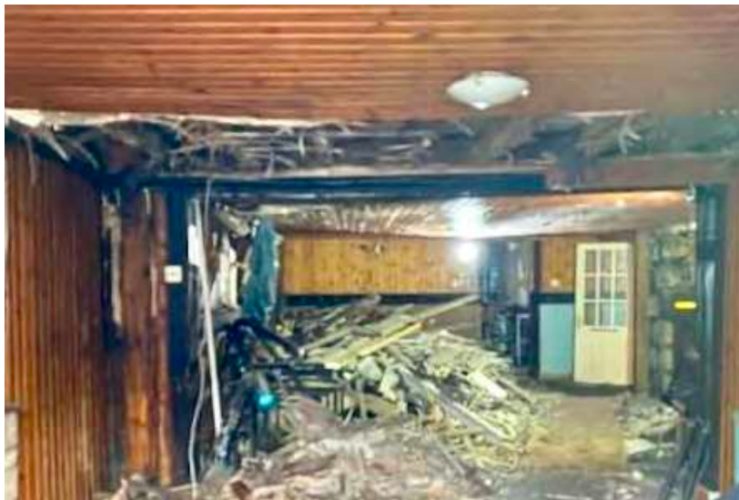
Renovation work on the Baird Centre, which is part of the old Dower Hotel.
